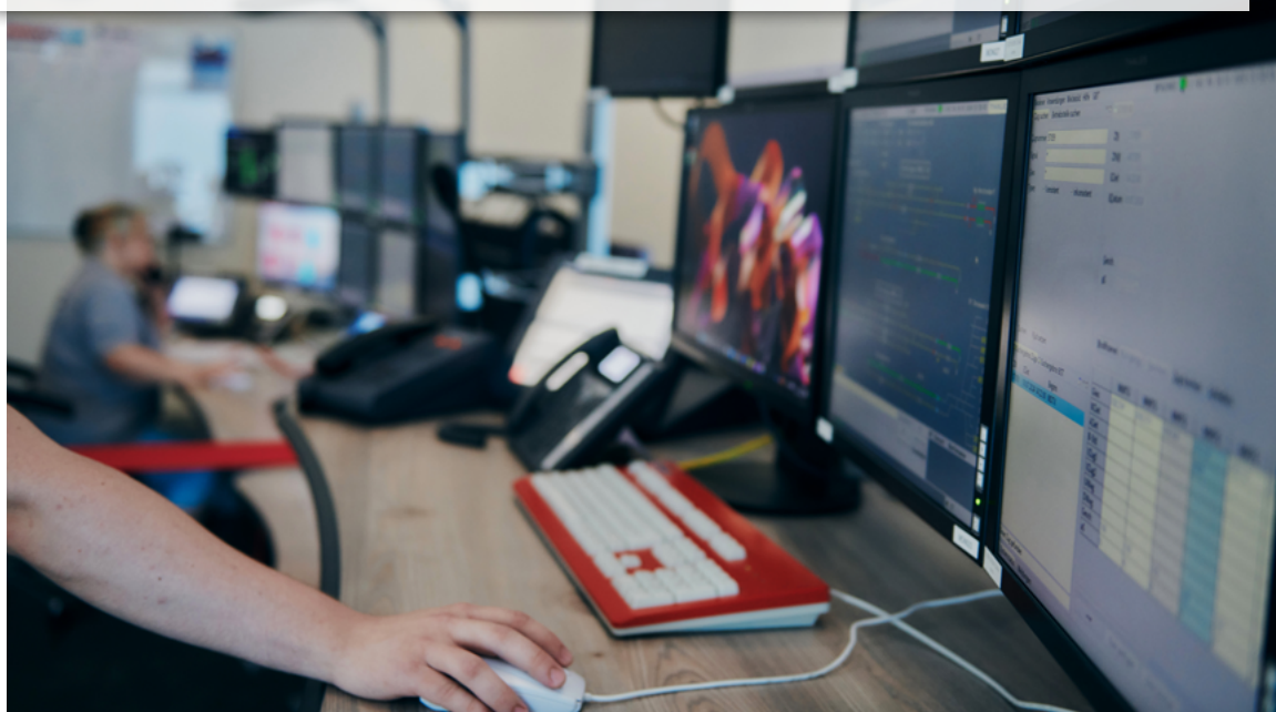
Central control interfaces in the Donauwörth digital signal box
