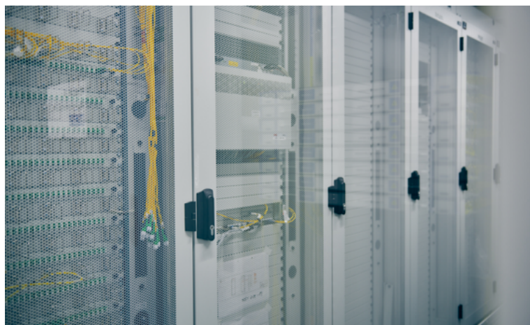
Server room in the Donauwörth digital signal box
